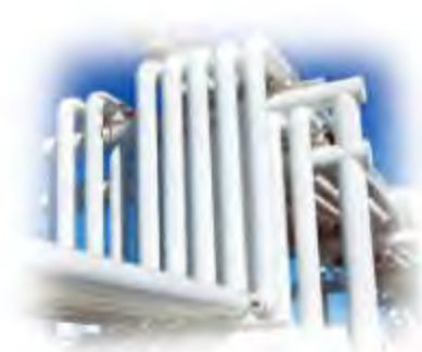
Industrial Gases Pipeline
