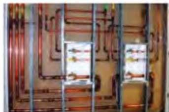
Medical Gas Pipeline
